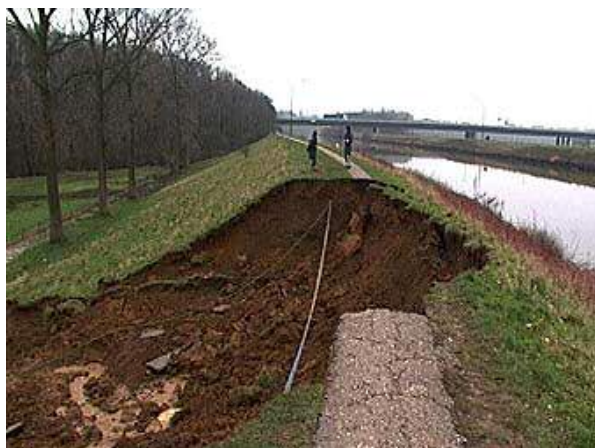
Fig. 8. Inner slope dike failure near Stein
