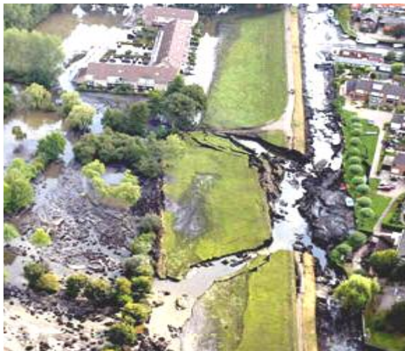
Fig. 2. Shifted part of a canal dike
